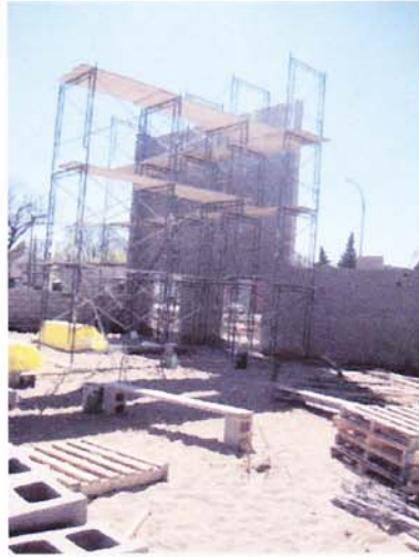
THE LAST OF THE EARLIER STAGES OF THE MASONRY WALL GOING UP
